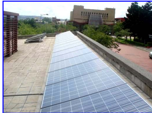
苗栗區農改場5.1 kWp
